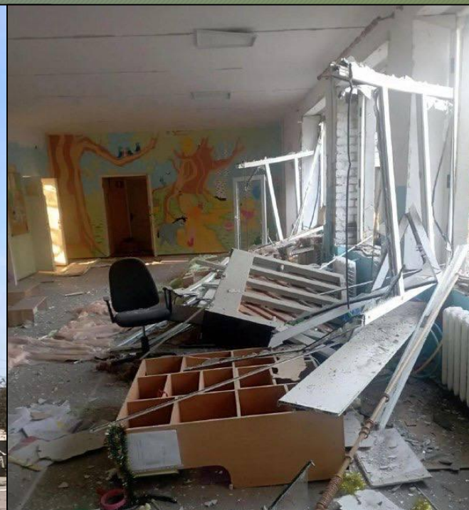
September 3 - a UAV strike on a kindergarten building in the village of Skelki, Zaporozhye Region.
