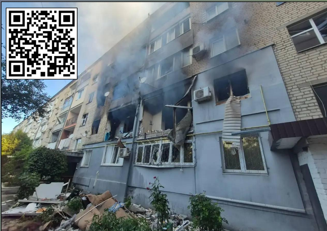
June 29 - a mortar strike on an apartment building in Kakhovka, Kherson Region. One civilian was wounded.
