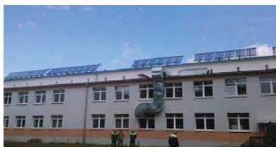
Solar collectors in machinery college in Vitebsk
