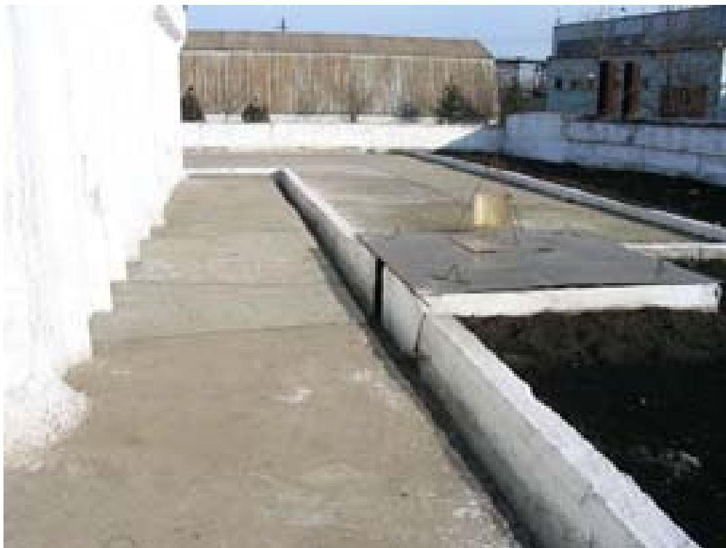
Figure 4: Rainwater drain system and sampling vault of the contaminated dust storage facility
