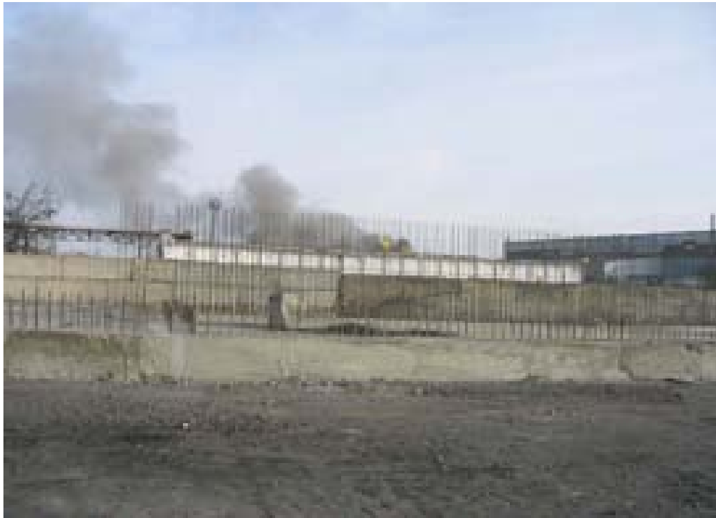
Figure 7: Construction of the new storage facility for contaminated dust from the source-melting event ( ^{137}\text{Cs} ) in 2003
