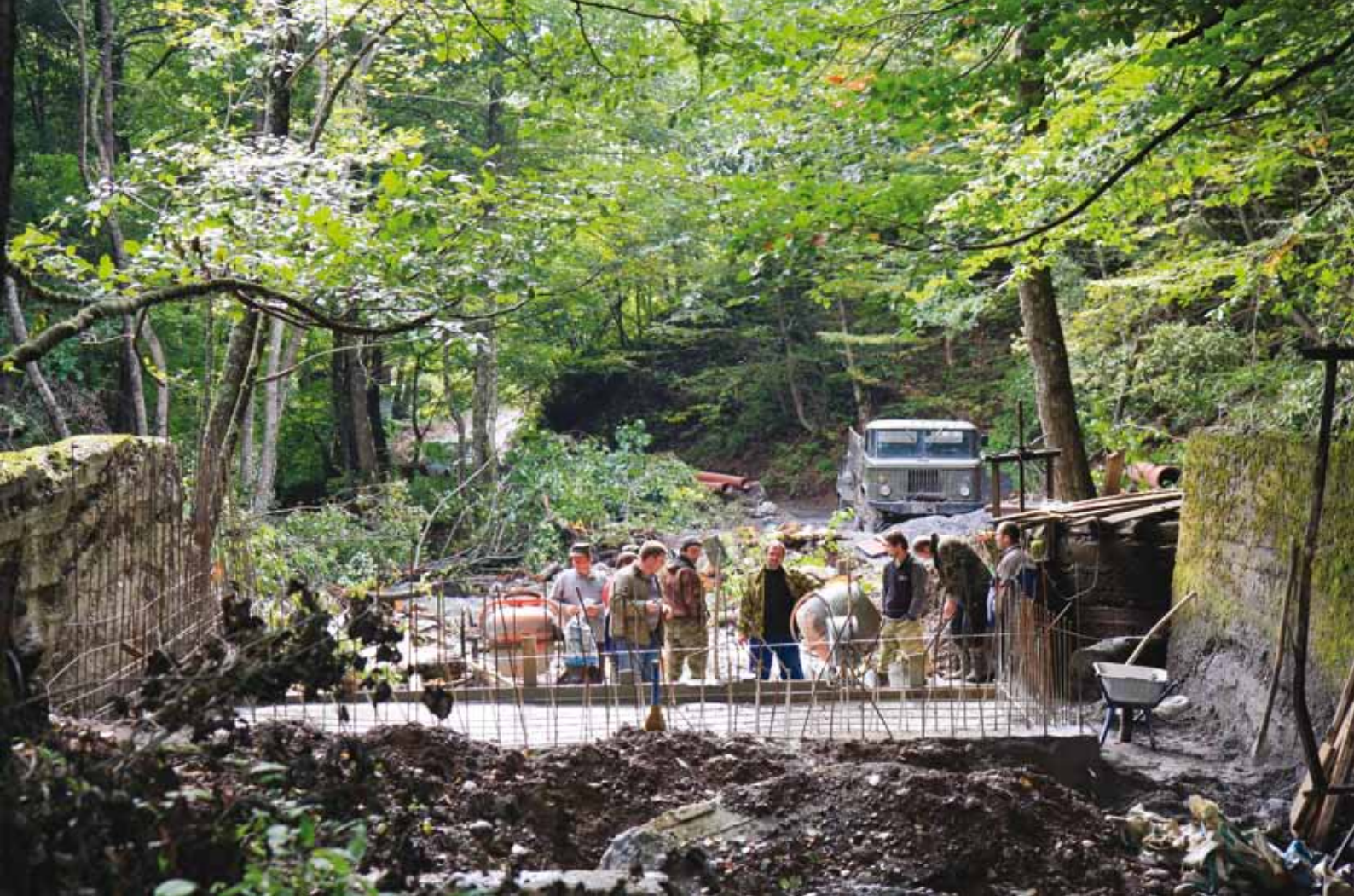
Repair work on the intake of the Znauri water distribution network, being rebuilt in an EU-funded OSCE project, managed by the CPC, to build confidence in the region affected by the August 2008 conflict in Georgia. From the intake, a nine-kilometre pipe will bring potable water to Znauri. (OSCE/Emmanuel Anquetil)
