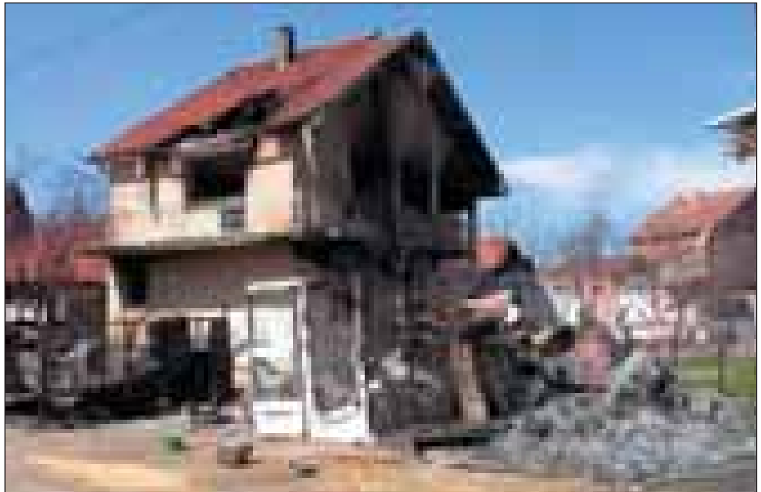
Destroyed building in Lipjan/Lipljan on March 18
