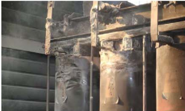
Figure 3.3. 10kv capacitor three-way reactor burnout and porcelain insulator burst in Guanghan Sanxingzhui substation
