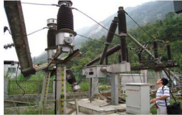
Figure 3.2. Most of transformers and circuit breakers are damaged in Beichuan 110kv Qimingxing substation
