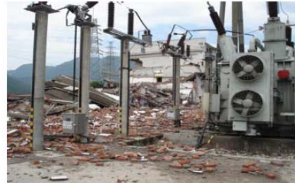
Figure 3.4. Main control room collapsed, transformer displaced and oil leaked
