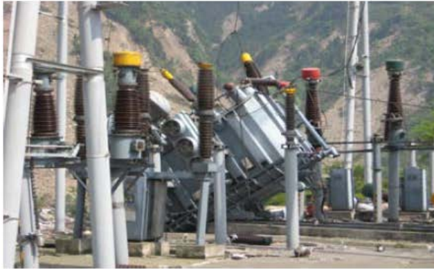
Figure 3.1. Transformer toppling down in 220kv Ertaiشان substation
